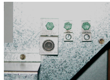
Required Ground Lug Installed
